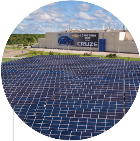
GM solar installation; Lordstown, OH.
